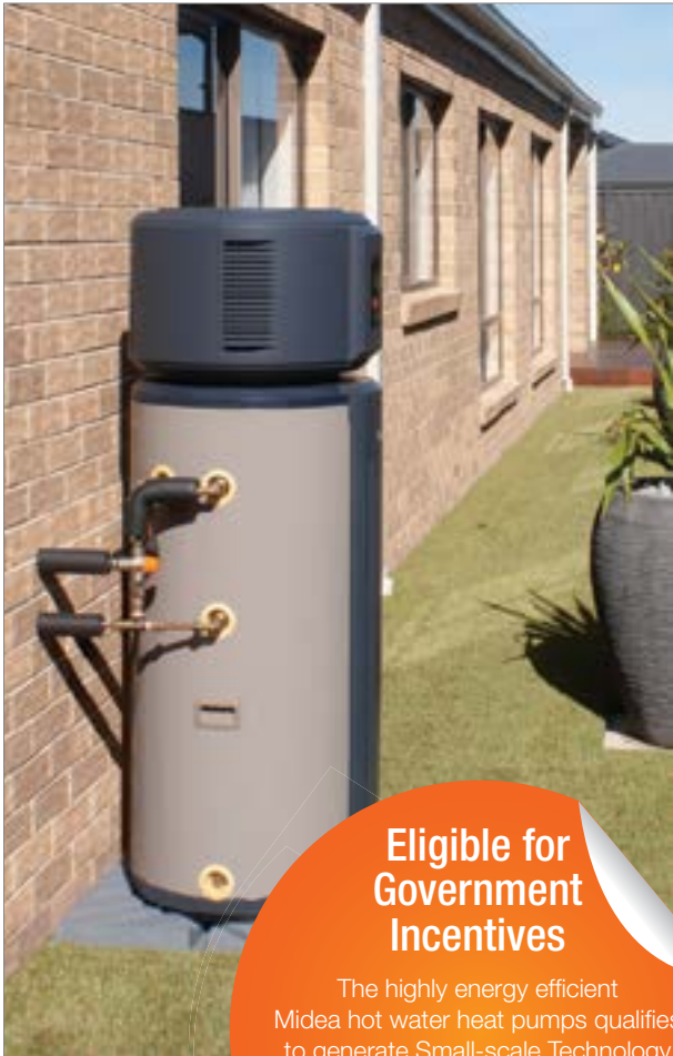
170L Installed Unit
